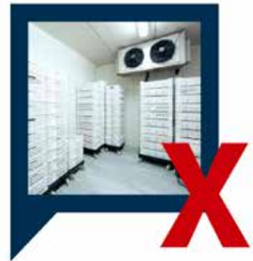
Cold storages (must not operate below 2 °C (35.6 °F))
